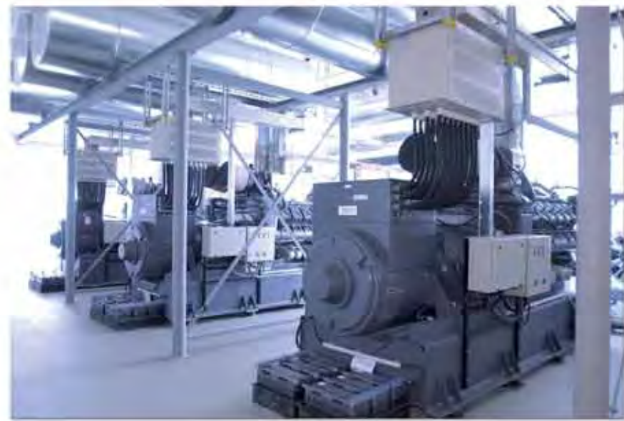
3 x 1650 kVA Aggregate
